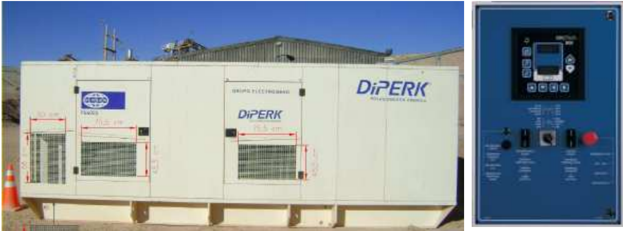
Figure 8.3-1: PE660 Genset and Synchronization Panel
